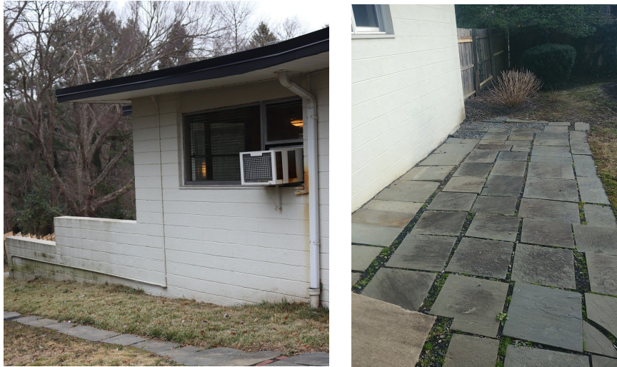
(L-R): Fig. 4.6: The only downspout located on the south elevation; Fig. 4.7: South corner of garage without downspout.
