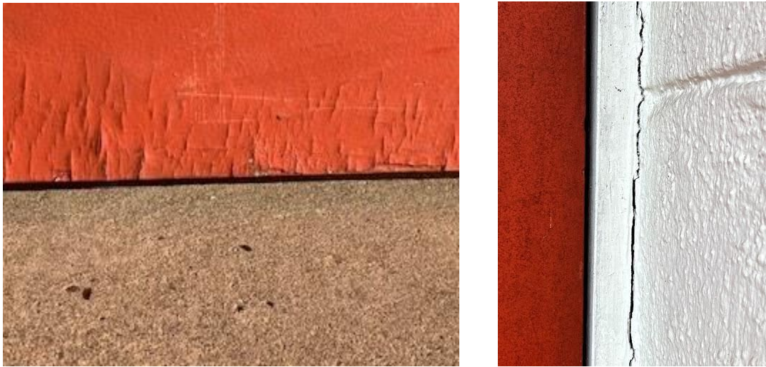
(L-R) Fig. 4.13: Peeling paint at bottom of red door. Fig. 4.14: Jamb of red door pulling from CMU wall..
