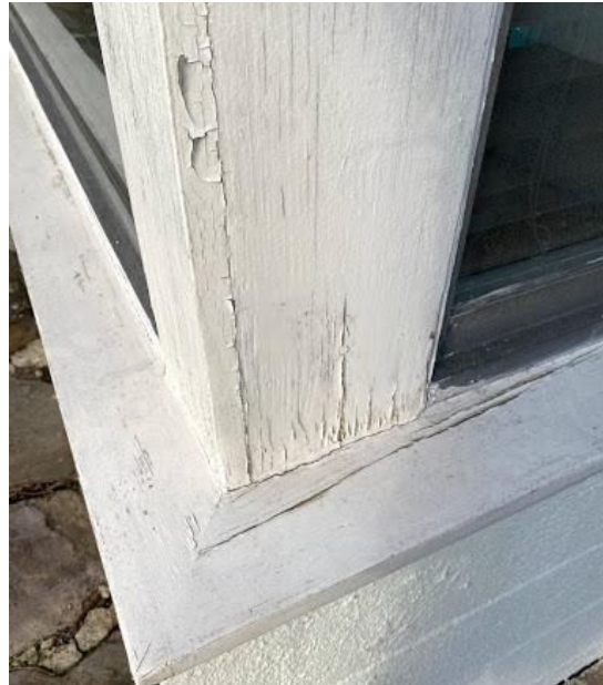
Fig. 4.16: Corner column on north elevation with cracking paint.
