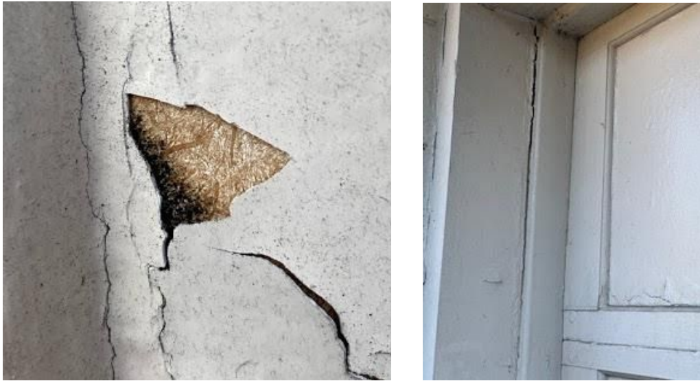
(L-R) Fig. 4.10: Exposure of OSB behind peeling paint. Fig. 4.11: Garage door trim peeling from wall.
