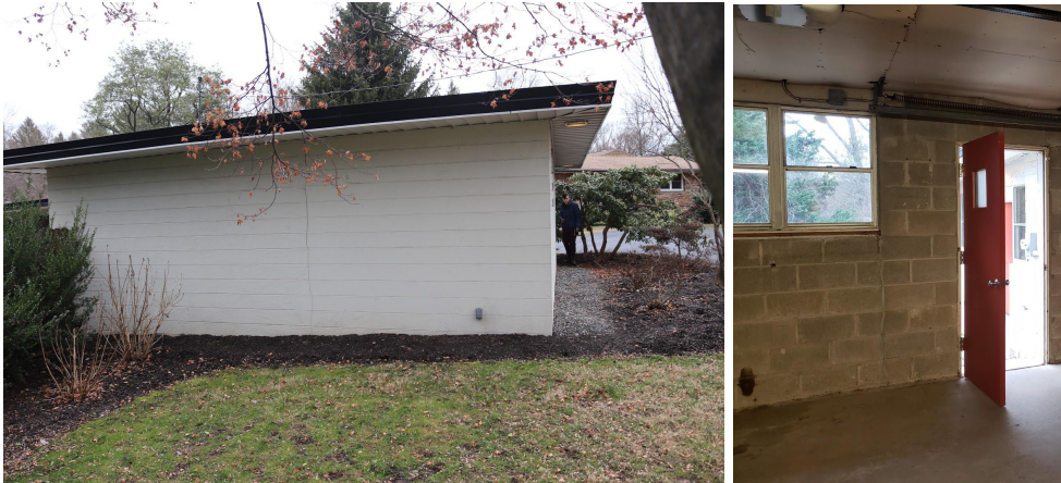
(L-R): Fig. 4.8: Active crack on the east elevation of the garage; Fig. 4.9: View of crack below window of garage.
