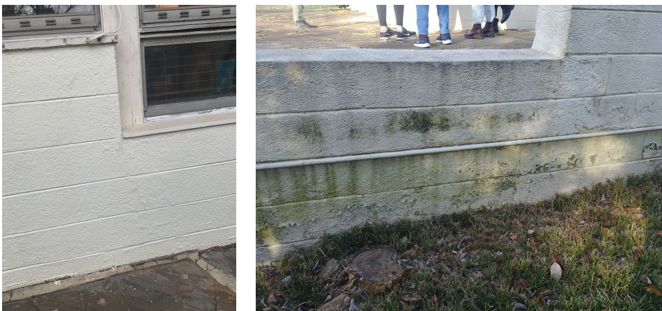
Fig. 4.1: Repaired crack on west elevation; Fig. 4.2: Algae on south elevation retaining wall.
