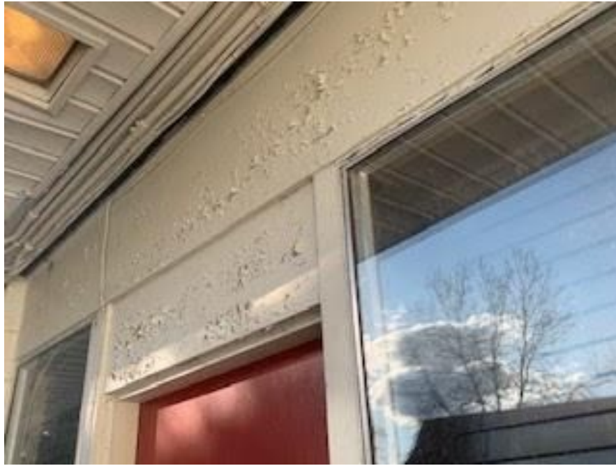
Fig. 4.15: Most severe peeling paint on the window and door panels of the west elevation.
