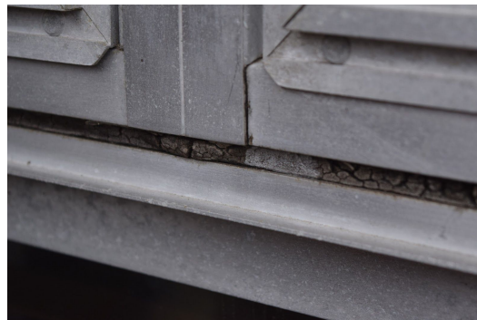
Fig. 4.18 Showing cracked gasket between frames.
