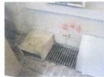
12 Existing HVAC in Greenhouse below window AD2.1
